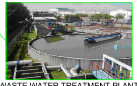
WASTE WATER TREATMENT PLANT 污水處理廠
